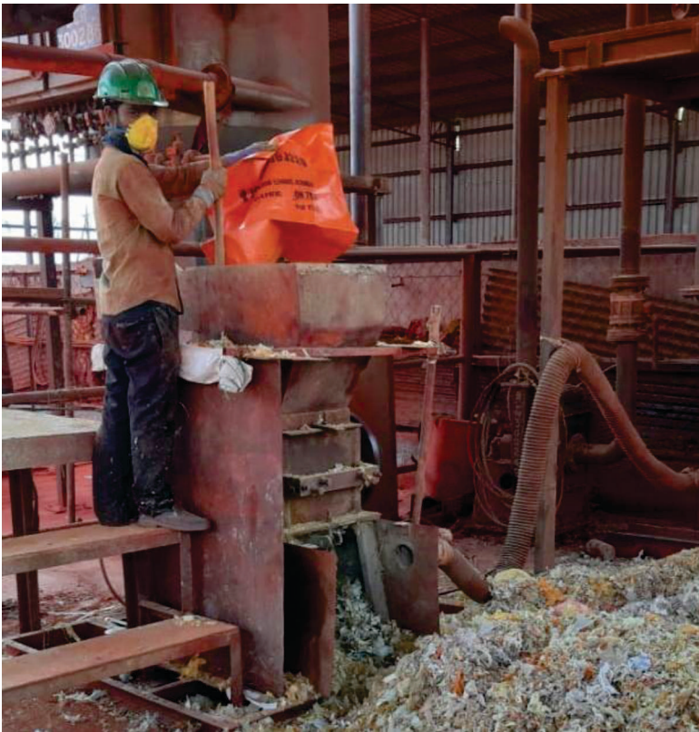
Plastic shredding machine installed at scrap yard
